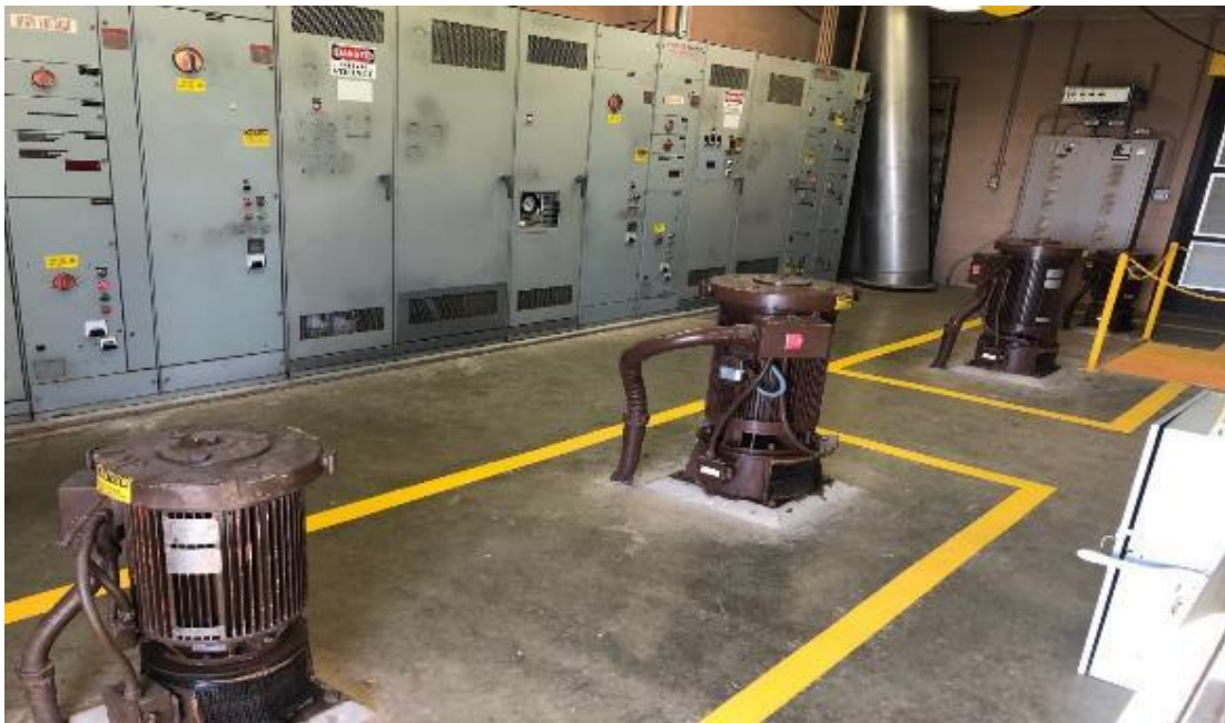
Photo 2: Interior West Side – Motor Control Center (MCC) & motors mounted on ground floor base which connects to pumps below in dry well.
